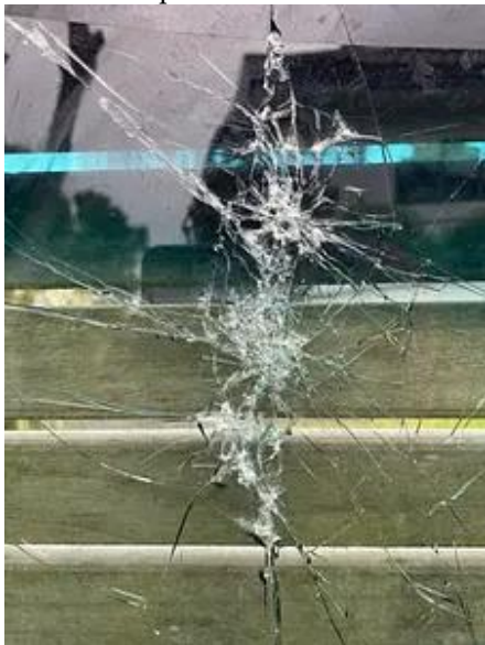
Figure 5. Spider cracks caused by striking.
